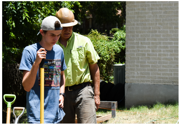
Heritage Junior, Josh Tabor, working with Mark Cornett to lay the foundation for a carport here at Mision De Candelilla!
