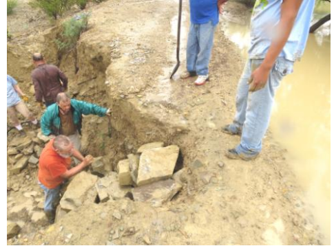
After we pulled Pastor Pepe's truck out we went to work. With great energy the group piles tons of rocks in the hole to give us safe passage. Everyone was soaked by a light rain that fell while we worked.
