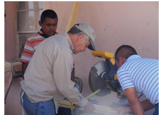
Carlos Servin is showing the guys from Las Norias how to do it. Carlos headed up the carpentry in February to screen all the windows and doors in the village. The project was funded by the Rotary District 5840 Hunger-plus Committee. While the group was working Sara Allerkamp and Juan Flores held VBS classes. Then at the evening worship services the kids would sing the songs they had learned during VBS classes.
